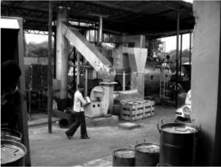
Figure A8.9 Boiler.
