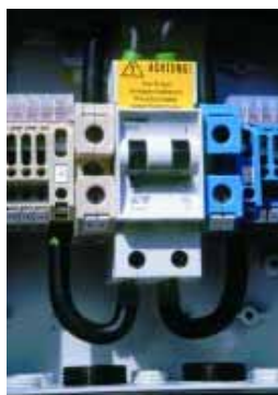
Figura 3.101 - Interruptor principal DC
