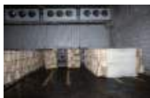
Figure 47. Commercial forced air cooling system.
